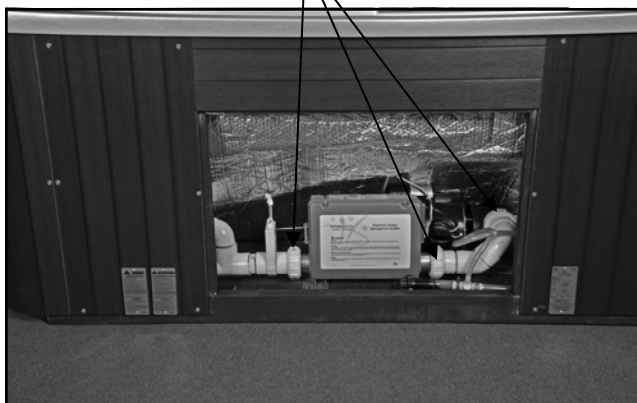
...THROUGH THE PUMP UNION
